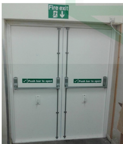
Figure: Double fire doors with door co-ordinator
