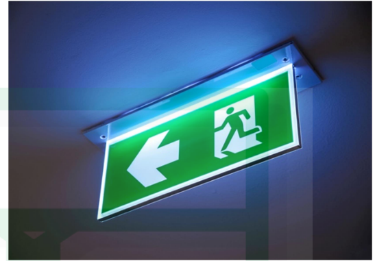
Figure: Emergency lighting built into Signage
