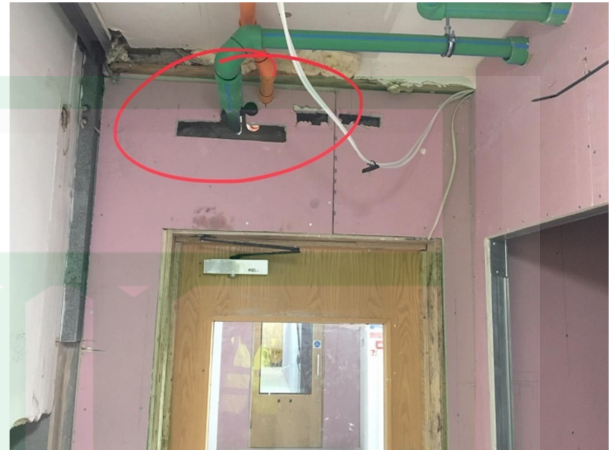
Figure: Poor fire stopping without penetration seals
