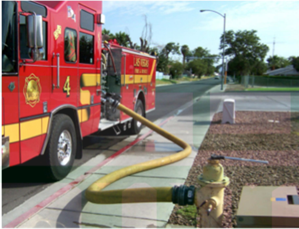
Image: Fire hydrant in use
