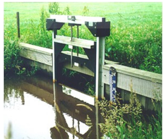
Picture Penstock which can be shut if there are any discharges which need to be stopped from entering the river
