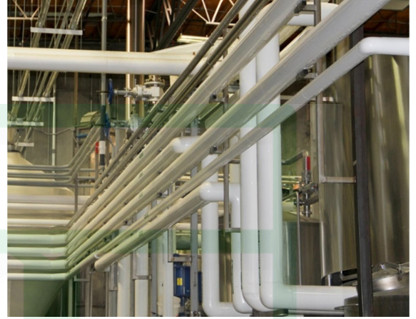
Piped gas supply
