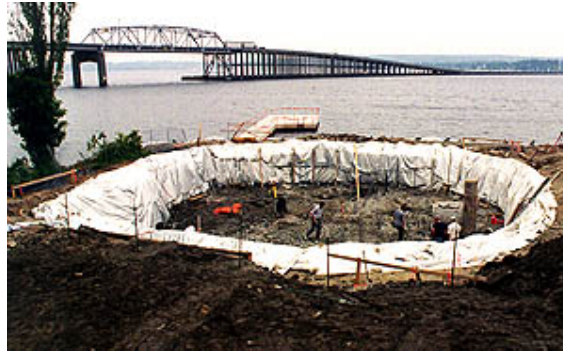
Frozen soil shoring for an access shaft at Bryn Mawr utility improvement project in Renton.
