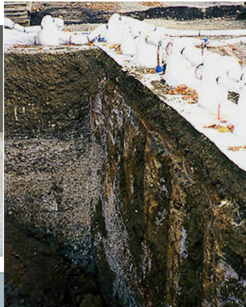
Frozen soil shoring wall around a 10-foot-deep basement excavation for a condominium in Madison Park.
