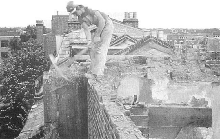
Picture: - Work at height has not always been well managed
