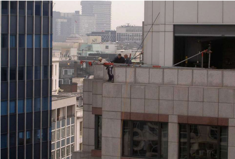
Picture A more modern example of poor working practices
